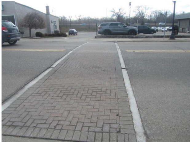
Figure 51: Crosswalk Condition Near Police Department Along Auburn
